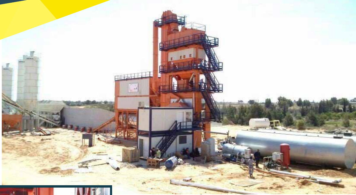
240 TON/HOUR ASPHALT PLANT - TRIPOLI/LIBYA 2011
